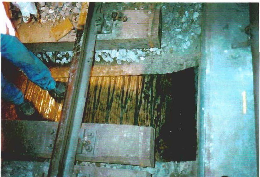
Fig. 4: Exposed area - visible is the lower SBM-layer
